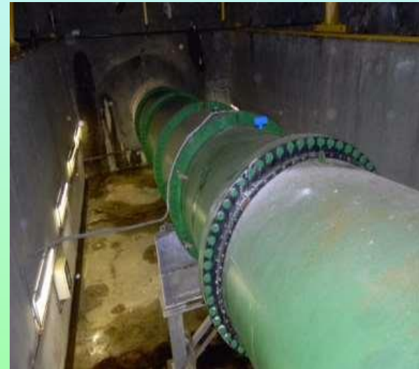
Flow measurement equipment
