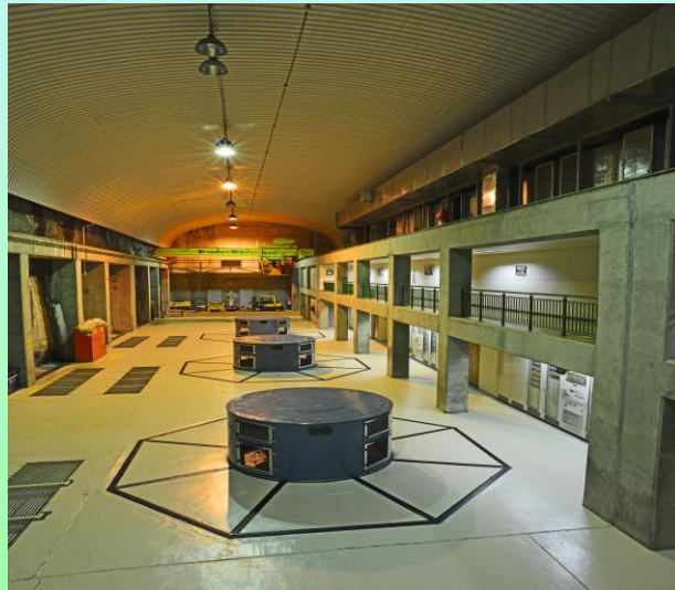
Muela Hydropower generation chamber
